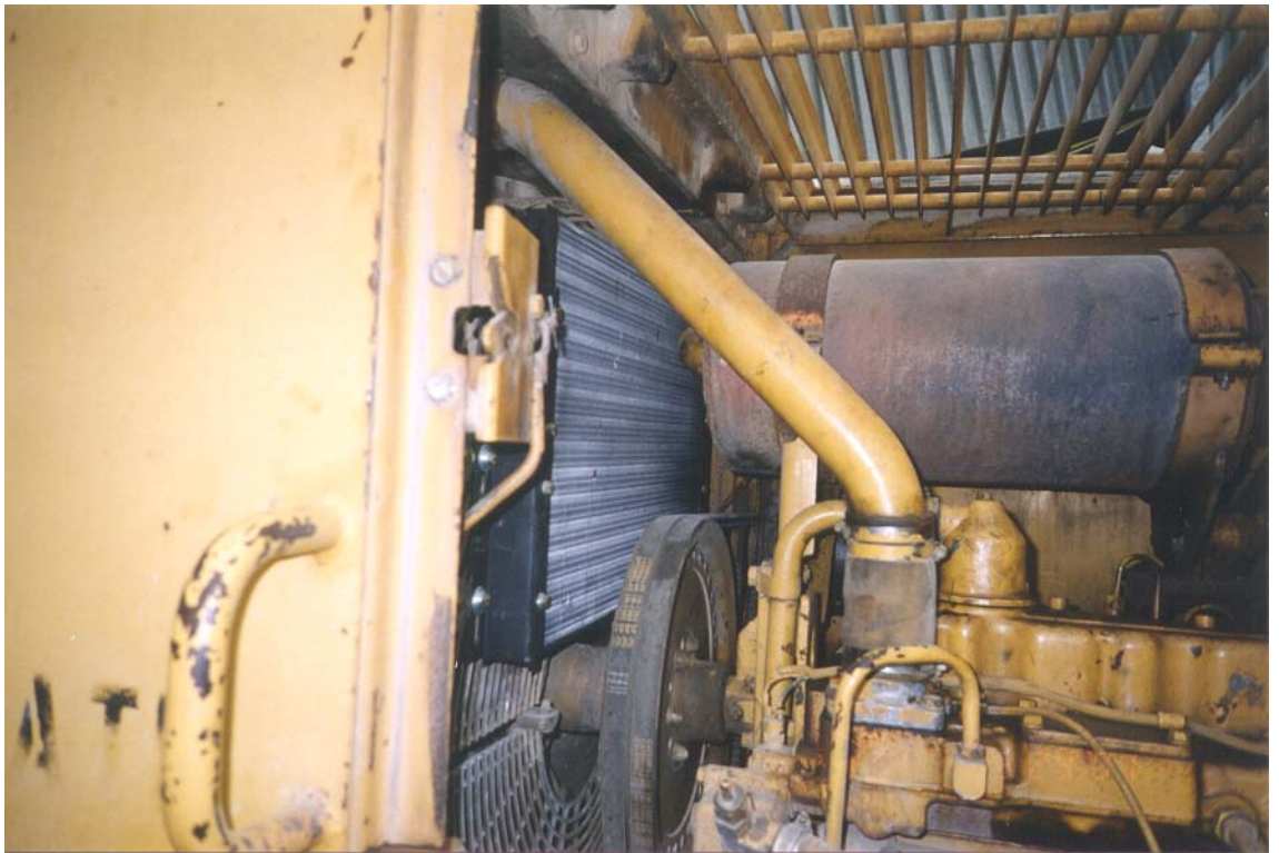
Condenser as viewed from right side.
