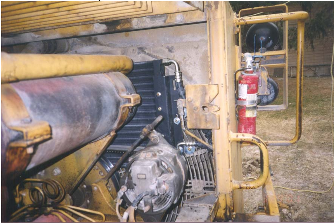
Condenser as viewed from left side.
